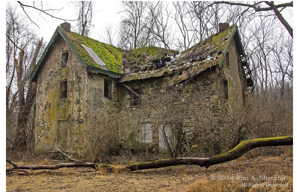
Exterior view of the Jacob Minshall dwelling house at Ridley Creek State Park. January 2014.
